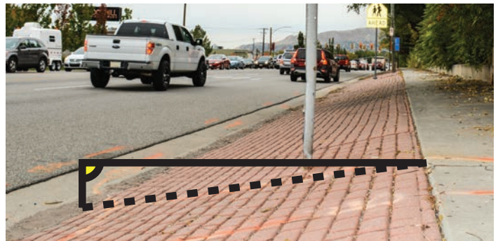
Foothill Drive has a number of narrow sidewalks with significant park strip slopes toward the street which present safety hazards for pedestrians and users with disabilities.
