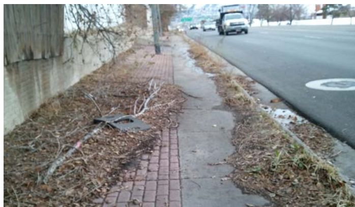
This section of sidewalk along Foothill Drive shows one example of a lack of maintenance.
